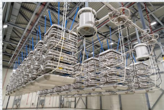
HVDC Light® NordLink (1,400 MW / ±525 kV)
